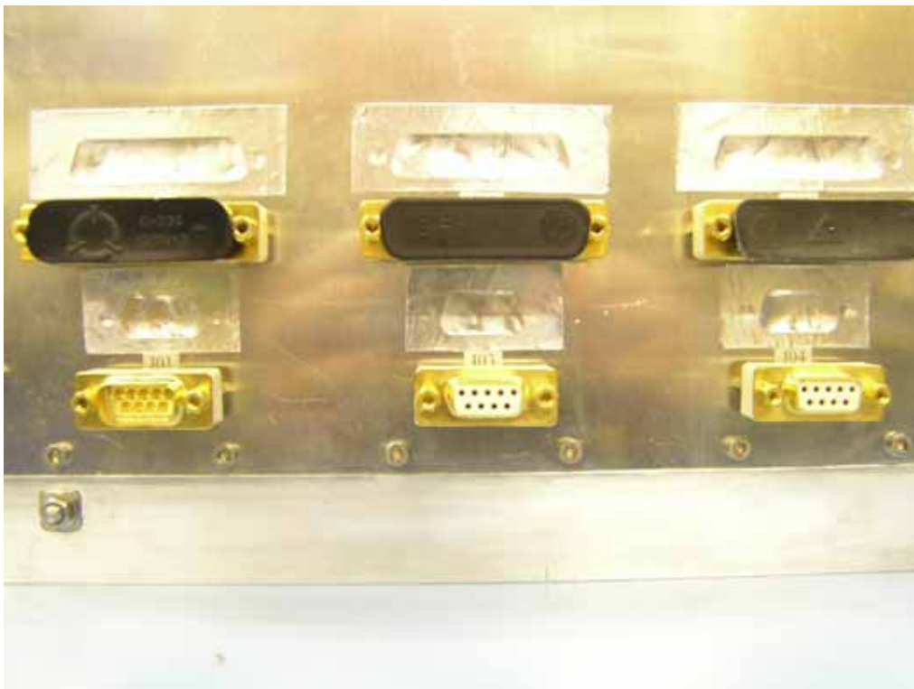
Front View showing connector savers fitted and 3 ESD covers fitted
