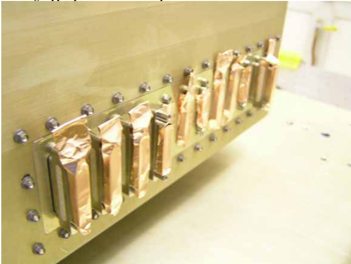
View showing copper protective covers in place and savers fitted to some connectors
