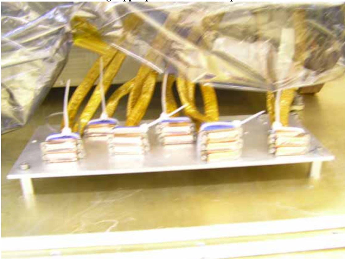
View of other Harness showing copper protective covers in place
