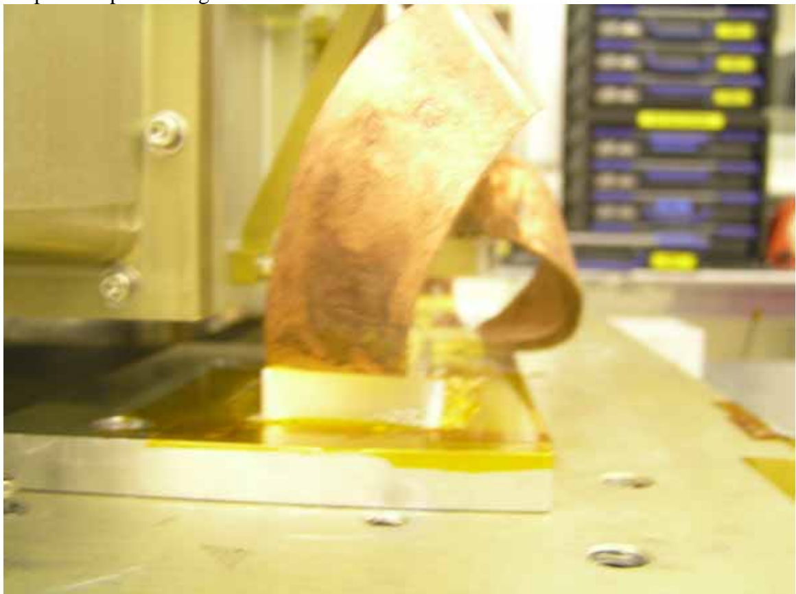
Close up of Straps showing discolouration
