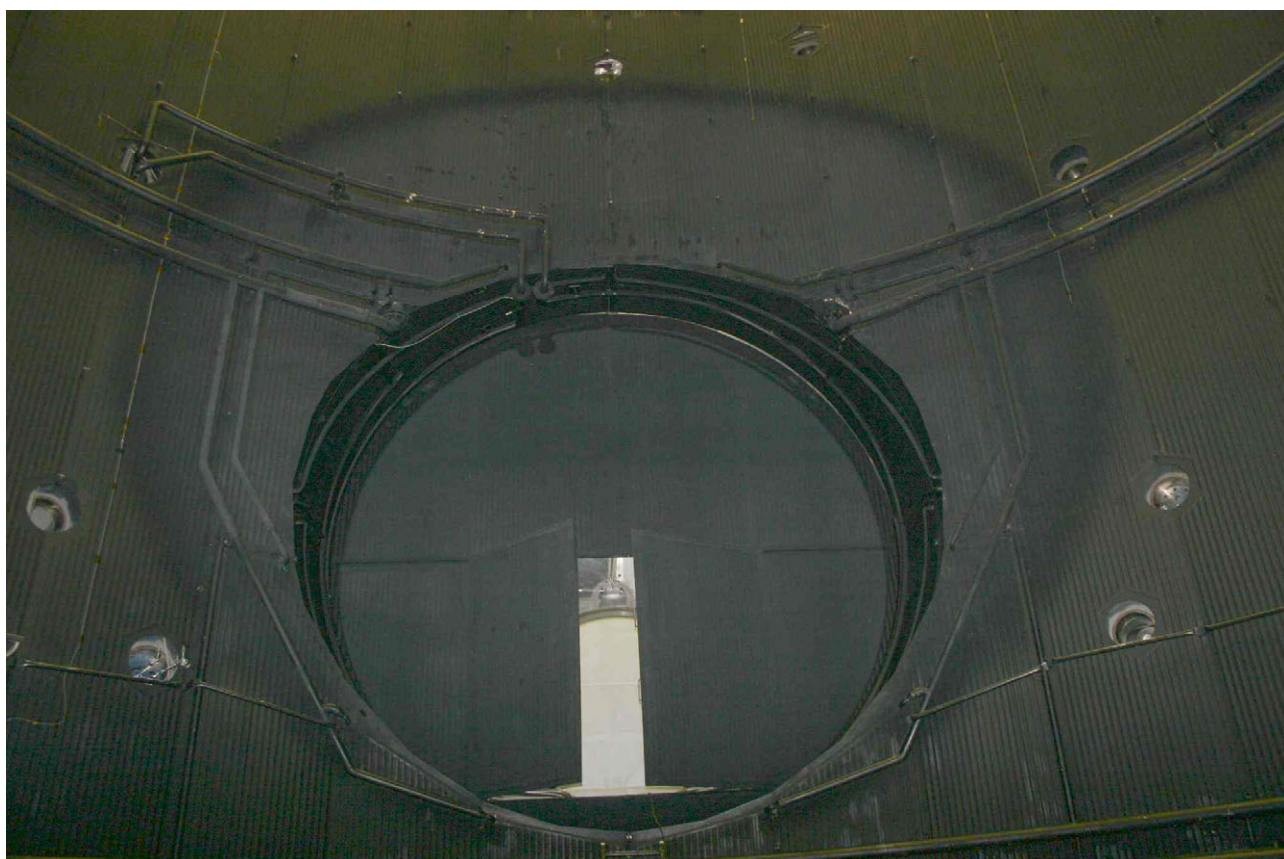
Figure 6.4-2: Sunburnt black surface of LSS back wall (SUSI switched off)
