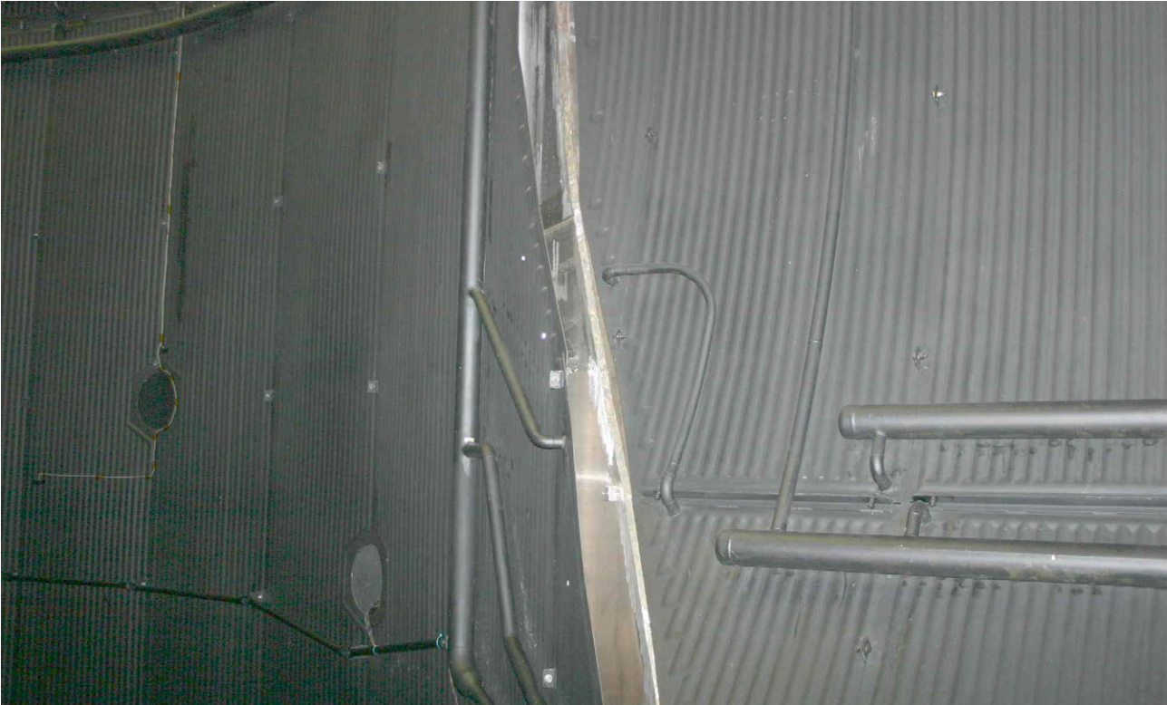
Figure 6.4-6: Circumferential gap in connection from nozzle to cylinder
